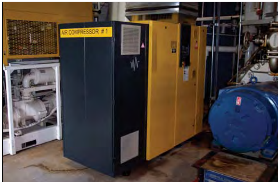
Picture of Milk Plant VSD Air Compressor
