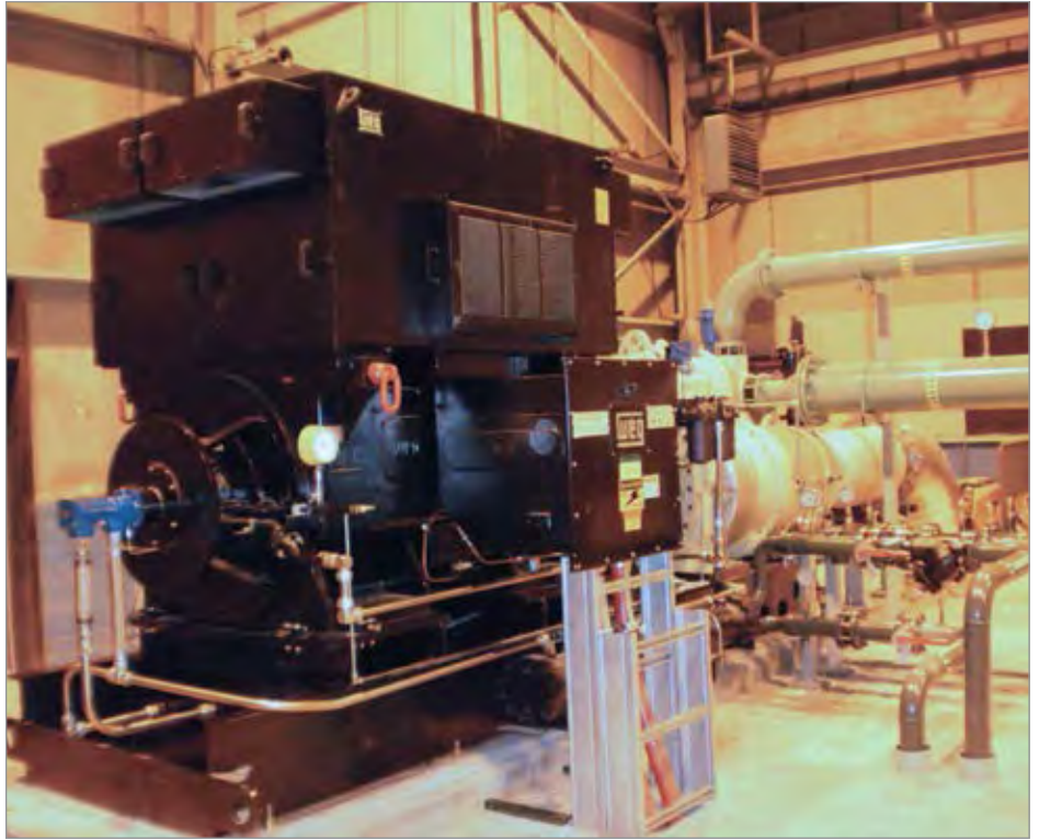
Figure 2: Replacing the old Turbo 5 with two new compressors has saved a significant repair bill, and has made the system more efficient.
