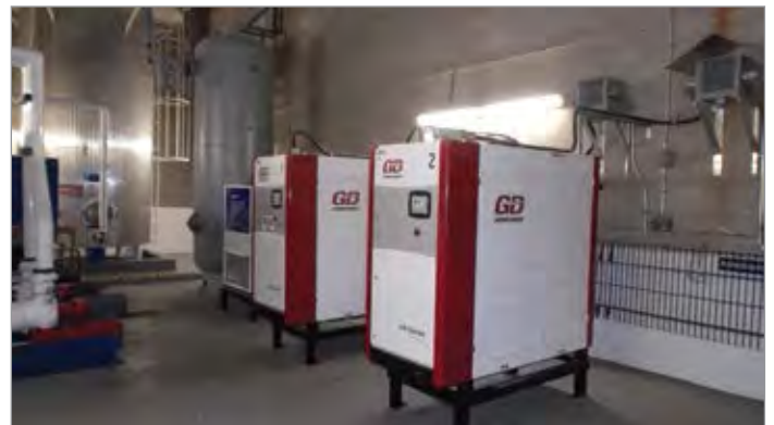
Figure 4: The new air-cooled compressors do not require an external cooler and heat an area of the plant displacing natural gas heat.
