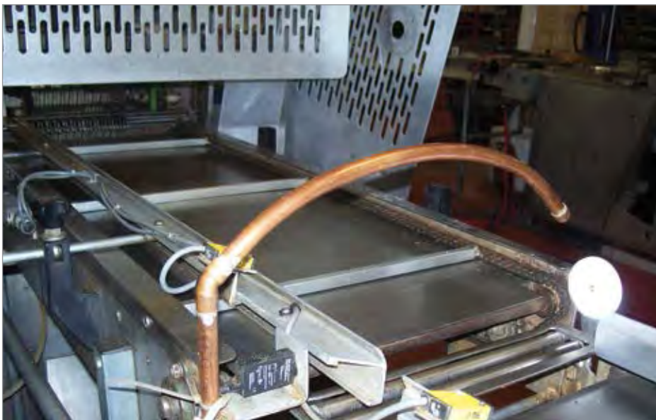
Figure 2: Typical locally designed blowing using copper tubing with holes drilled in it consumes expensive compressed air when other, more economical methods could be used.
